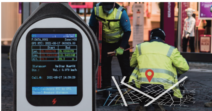
Locate noise source with GPS
