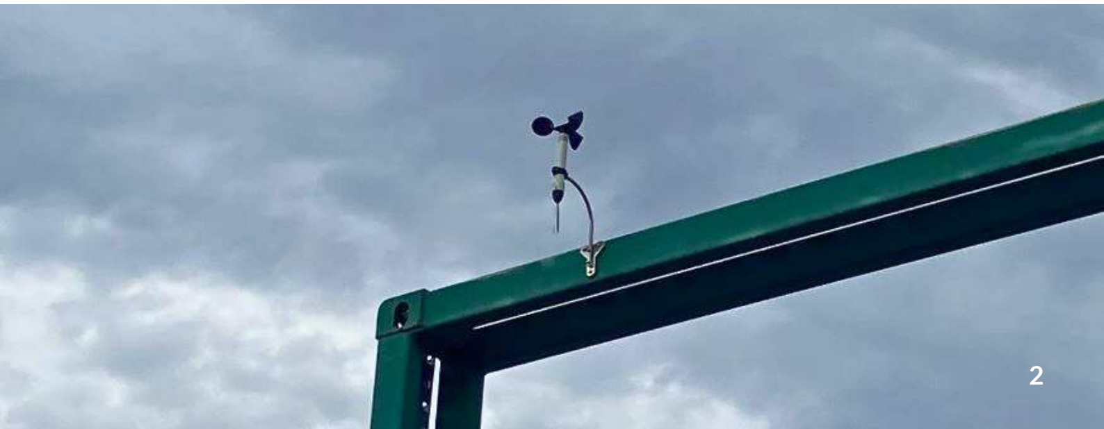
▼ WindPro wind sensor installed in empty container yards
